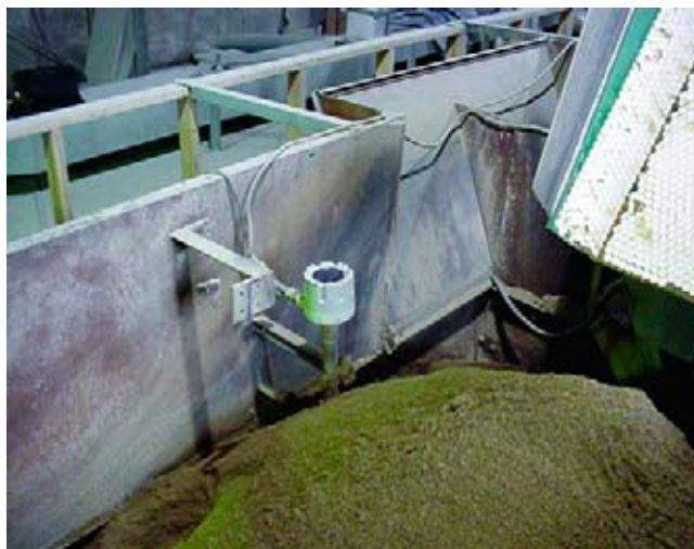
This rotary paddle bin level indicator has been mounted on an extension to detect high levels of sand in a bin at a concrete batch plant.
