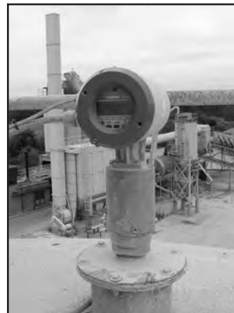
Flexar® technology on cement powder silo at concrete batch plant
