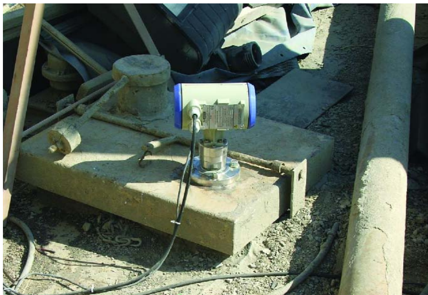
The continuous level sensor's electronics, which are protected by a NEMA 4X (IP66) aluminum housing, are installed on top of a silo.
