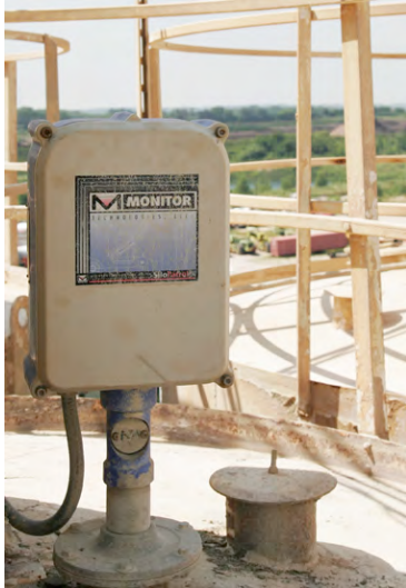
Figure 2. SiloPatrol ® weight and cable level system on top of a raw material silo.
