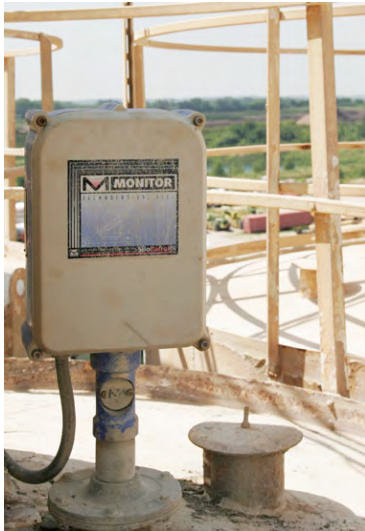
Figure 2. SiloPatrol ® weight and cable level system on top of a raw material silo.
